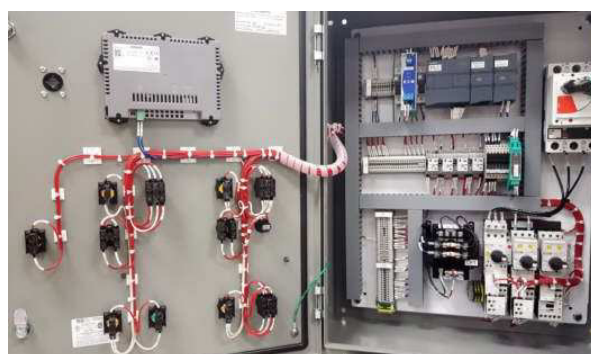
Fig. 4. Control system with PLC placed inside the rack cabinet with DIN rails
