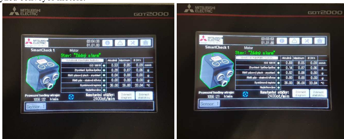
Fig. 8. HMI of Motor 1 and Motor 2 measurements
