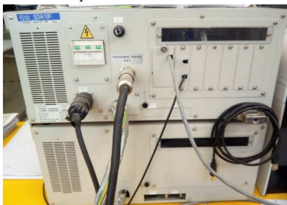
Fig. 3. FS 100 control system
