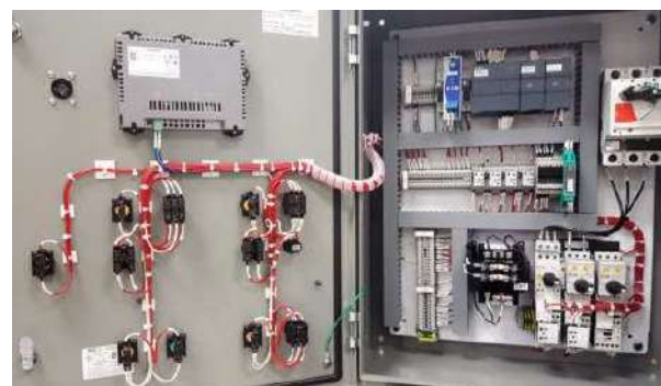
Fig. 4. Control system with PLC placed inside the rack cabinet with DIN rails
