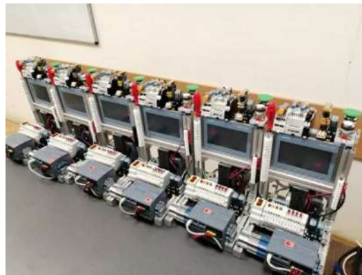
Fig. 11. Fully equipped training stands with programmable logic controllers
