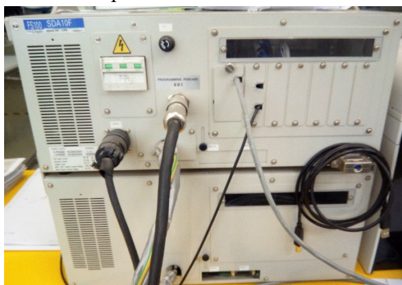
Fig. 3. FS 100 control system
