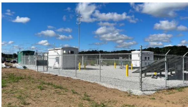
Fig. 2. Meter stations that measure the amount of gas being transported
