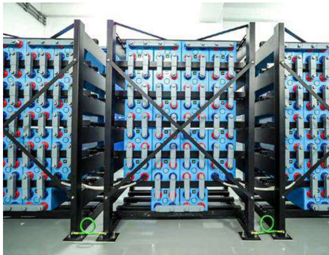
Fig. 4. Wellington battery energy storage system (BESS)
