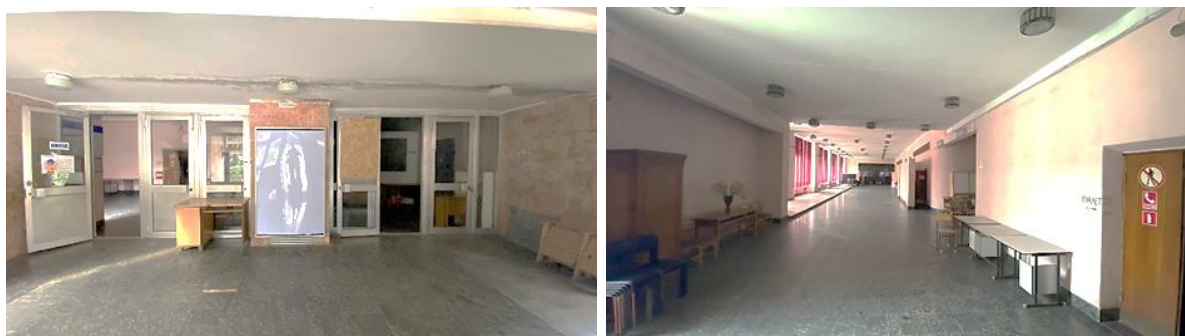
Fig. 3. Photo of the entrance and the perspective of the lobby of the «Peremoha» cinema
