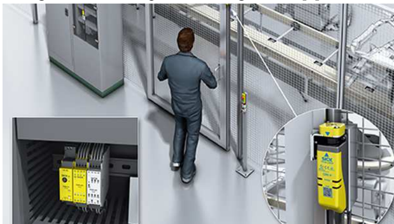
Fig. 4. Safety guards at automated workplace
